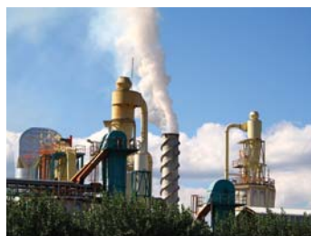
Steam exhaust from power plants
